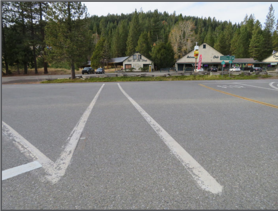
Figure 4.15: Intersection of SR 36 and SR 172 in Mineral needs crosswalks and re-stripping.
