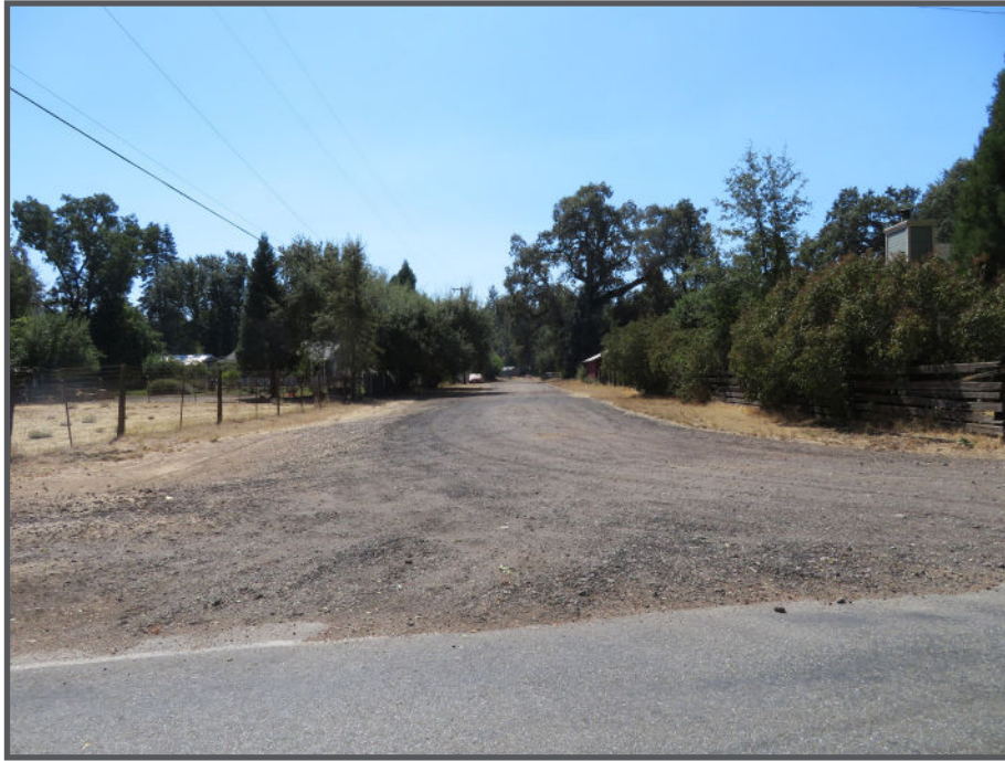
Figure 4.19: Unpaved streets in rural communities pose challenges to walking, biking, and people with disabilities.
